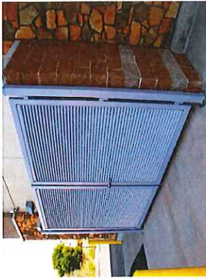
alum louver gate example installed in front of wall
